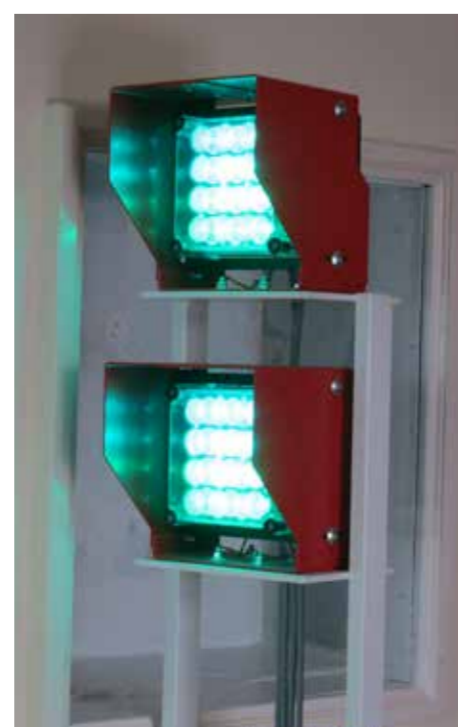
The ekta™ E8553 dual range lights installed in 2010 illuminating the green sector, photo V. Laitus
