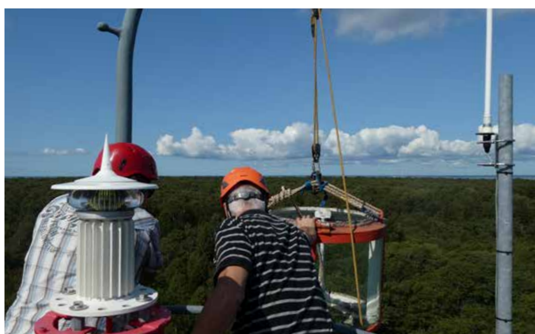
Routine maintenance in the Abruca Lighthouse in the year 2018 with the current LED-lantern in the foreground, photo T.Vilu
